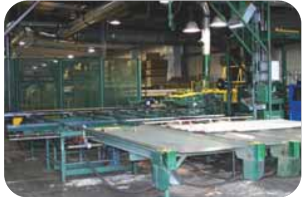
A Mid-Oregon International top arbor rip saw with six saws rips planed lumber to width.
